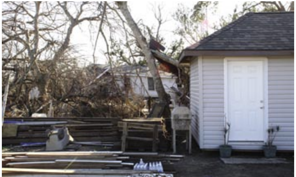
Buras, LA, February 4, 2006—A newly built shed is the beginning of one Buras resident's rebuilding effort. With assistance from FEMA she plans to completely rebuild her house in the same location, this time elevating the structure by 15 feet. (photo by Robert Kaufmann/FEMA)
