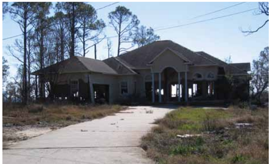
The unobstructed view through this home's entryway illustrates the destructive power of hurricane storm surges.
