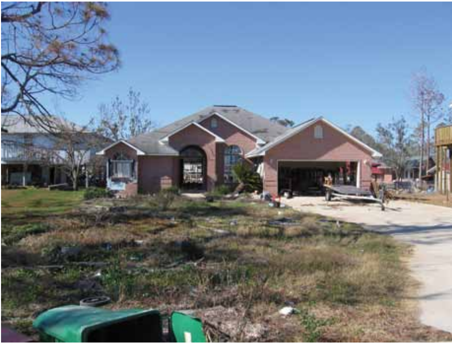
The fronts of homes did not always reveal the extensive damage behind and within the house.
