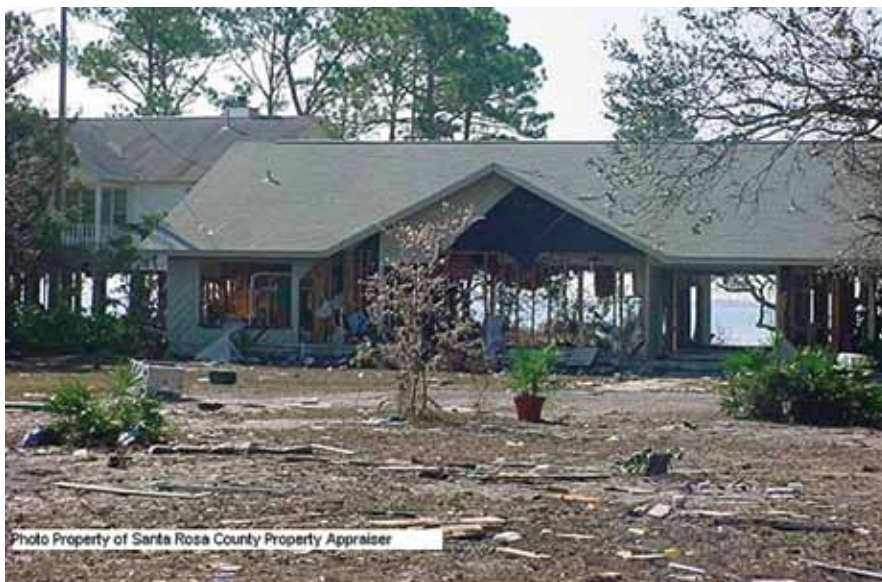
Homes with more than 50% structural damage are deemed total losses and must be rebuilt to new building code standards.
